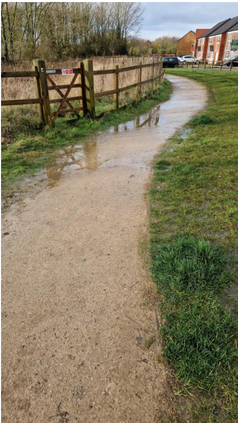
Photo 3 – Nothing to rectify the issues on this part of the path to the North of Coldham Grove entrance.
