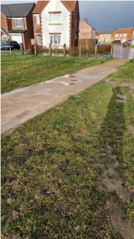
Photo 2 – Same issue on the path leading in from Coldham Grove.
